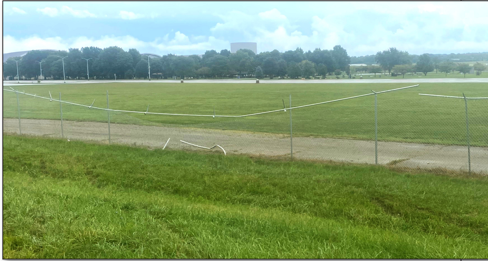
September 2022 damage to Air Force Base fence.
